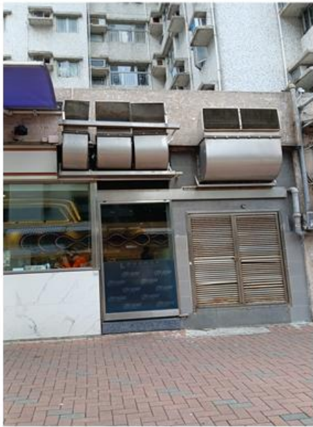
Figure 1: Spray oily vapour to pedestrians
